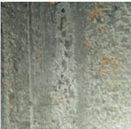
Fig. 1b Clearly visible in the close-up view: The corroded bearing material
